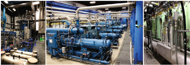
Fig. 2. Elements of the FRIB cryogenic system: (left) 4.5-K cold box, (middle) warm compressor, (right) tunnel transfer lines.
