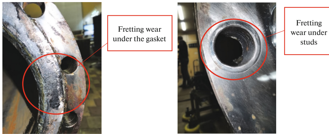
Fig. 5. Photographs of the inner and outer contact surfaces of the flanges after testing.
