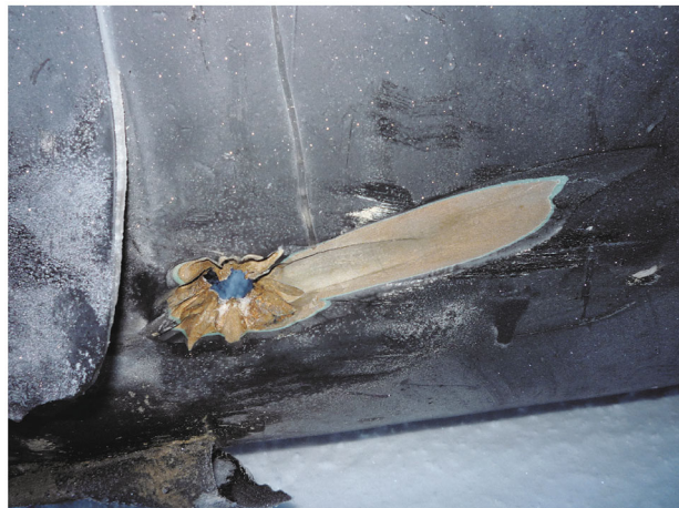
Fig. 3. Scab on the outer surface of a pipe.
