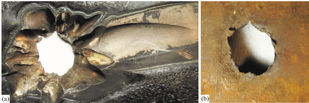
Fig. 4. Failed pipe: scab on external surface (a) and hole penetrating the wall to the inner surface (b).
