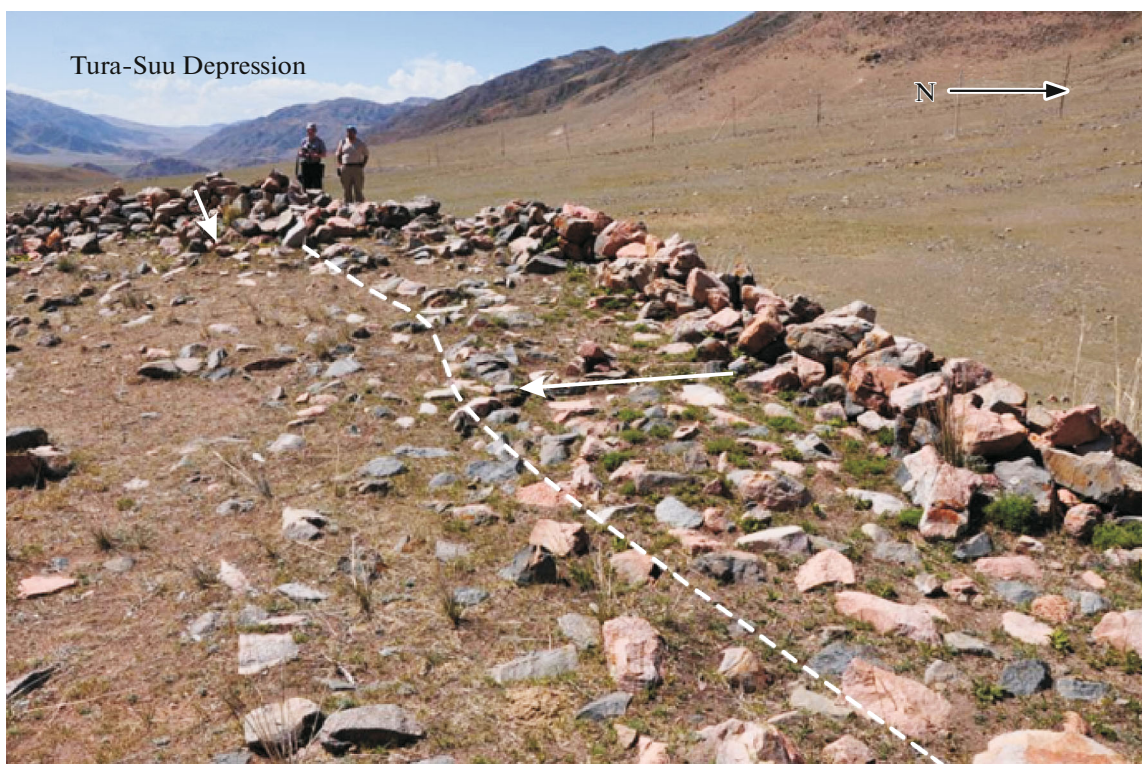
Fig. 5. Southern collapse of northern wall of Alabash Fortress (shown by long arrow). Dashed line, fragments of upper part of wall formed when it hit the ground. Western wall collapsed eastward (shown by short arrow). West view (after (Korzhenkov et al., 2018a), with changes).
