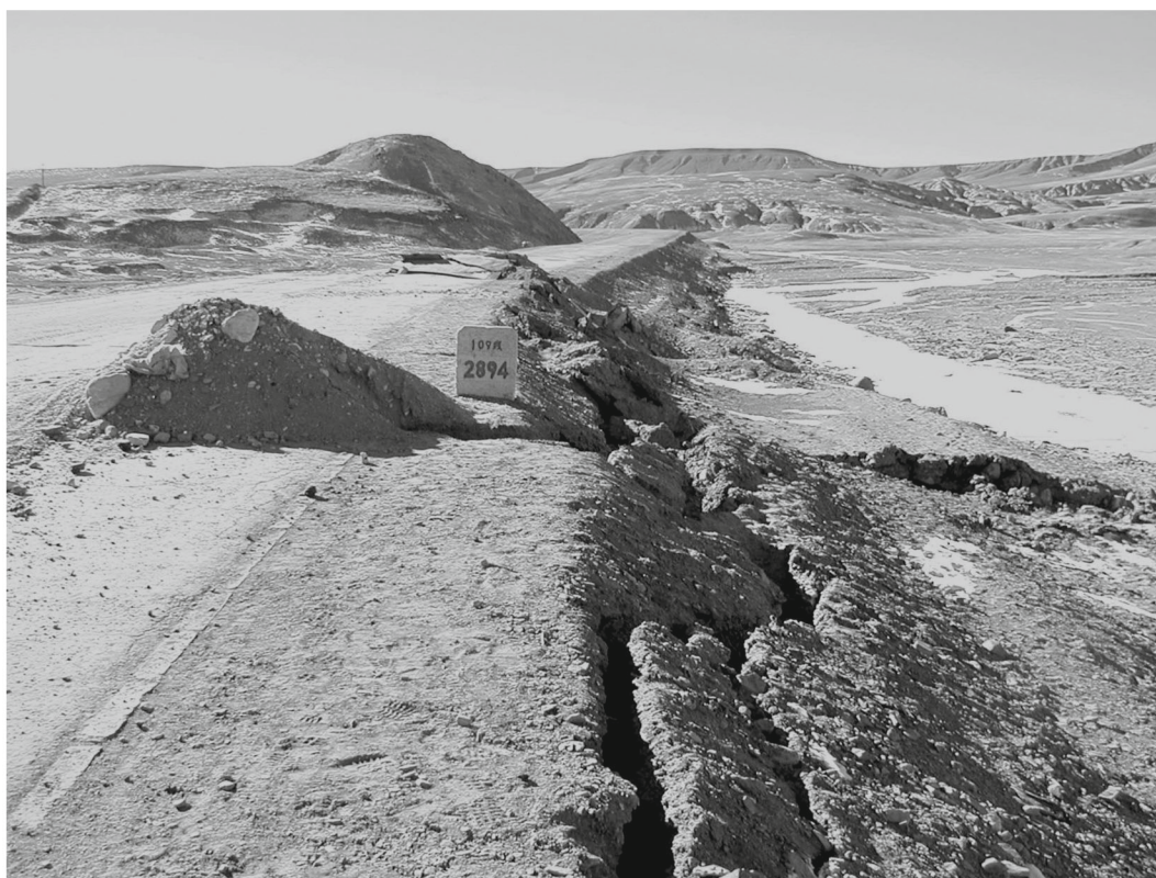
Fig. 5. Road damage caused by 2001 Kunlun earthquake. Photo by Jun Shen.
