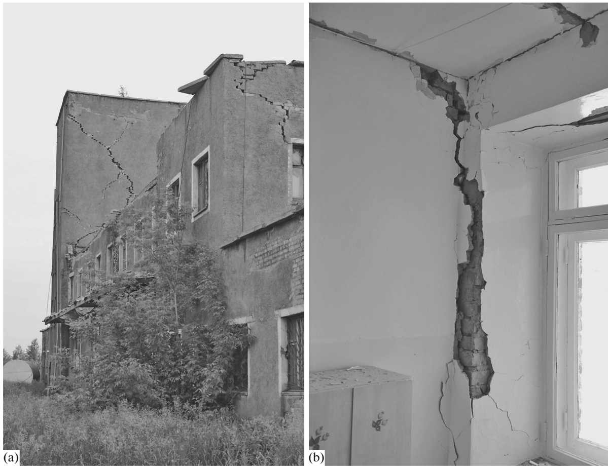
Fig. 3. Destruction of buildings during Bachat earthquake (village of Bachatskii, 4 km from epicenter).
