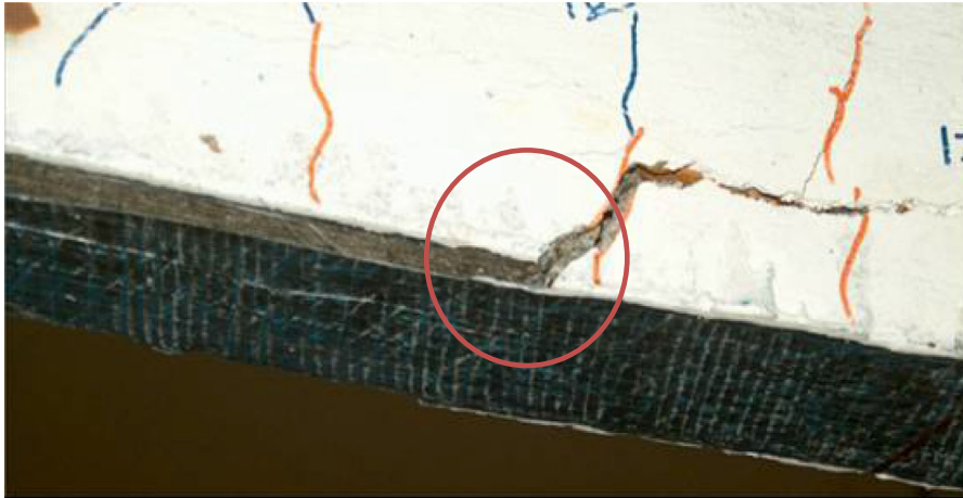
Fig. 13 Separation of concrete cover and CFRP in beam BS7.5
