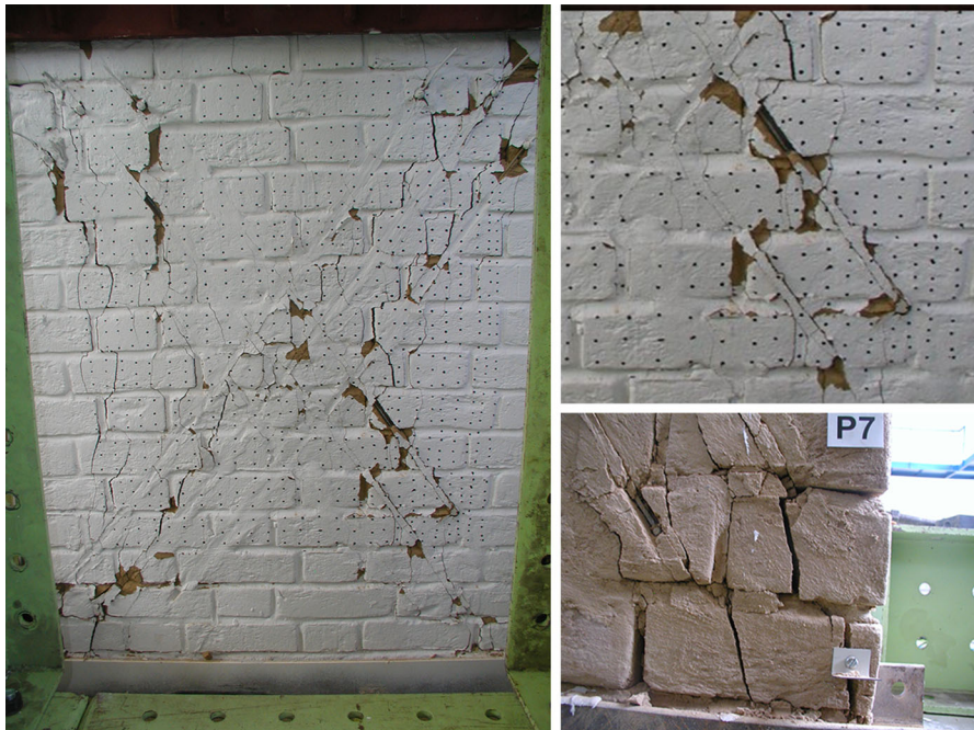
Fig. 11 Crack pattern (left), the out-of-plane deviation of the steel wire ropes (top right) and the damage of the corner (bottom right) near the rope anchor of a strengthened adobe brick wall
