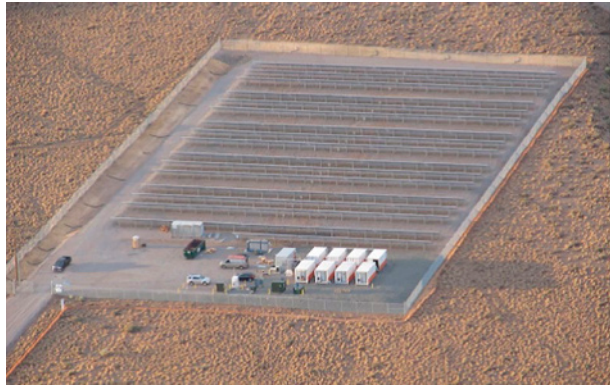
Figure 2. Aerial view of the Prosperity Electricity Storage Project in New Mexico, USA 56 (reprinted with permission).
