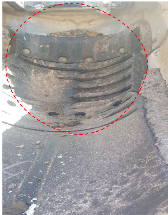
Fig. 2 Worn-out coating state
