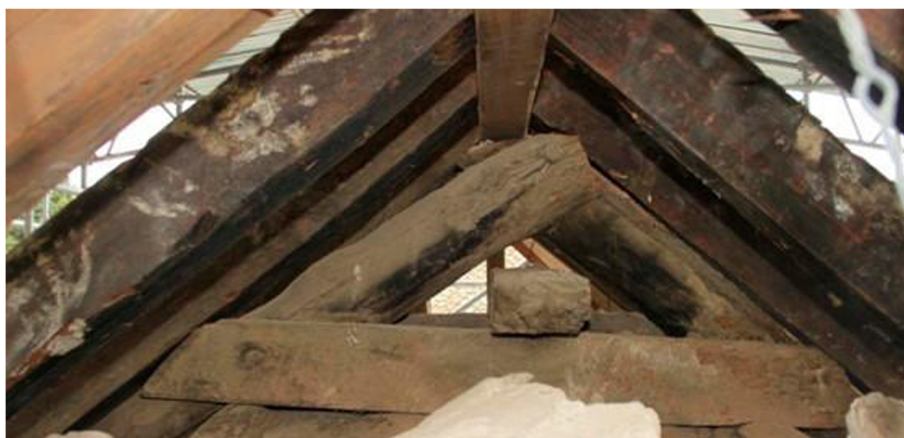
Fig. 16 Some rafters and a double false collar tie from the original Nasrid roof structure preserved beneath the upper roof structure built by Leopoldo Torres Balbás during his 1930 restoration (Source: Artyco 2015)
