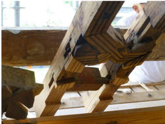
Fig. 15 Lower end of the rafters on the N-E slope, including the reintegration of the missing parts with new assembled insertions. This node illustrates the sophisticated and distinctive techniques of Nasrid carpentry compared to Christian- mudéjar carpentry (Source: Artyco 2015)
