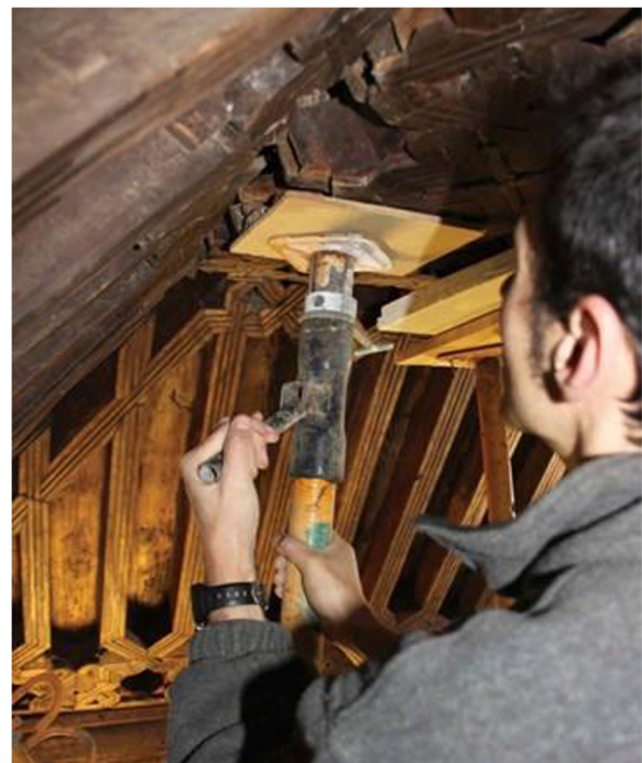
Fig. 14 Recovery of the structural deformations in the decorated timber framework using a mechanical jack (Source: Artyco 2015)
