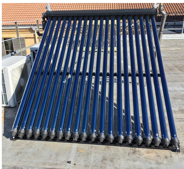
Fig. 3 The 20 evacuated tubed collector unit installed onto the roof
