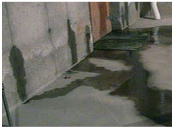
Picture Showing Groundwater Seepage through Cracks on Walls
