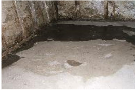
Picture Showing Groundwater Seepage through Building Floor
