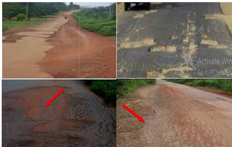
Fig. 2 Showing road failure in the study location
