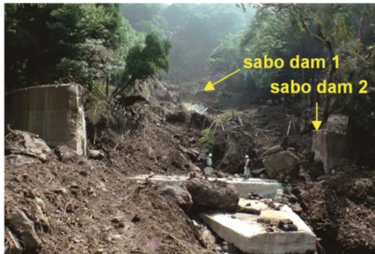
Fig. 12 Sabo dams destroyed by debris flow
