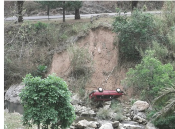
Figure 5 Some of the casualties of the Obudu landslide were the occupants of a car that tumbled when a slope near the road failed (photo by Igwe).
