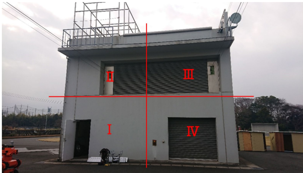
Fig. 9 Area that is divided into four sections on one side of the building
