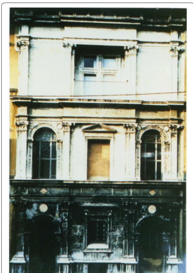
Fig. 8 The facade of the building in Bergamo (Italy) in 1993, before the conservation work [86], copyright (1996) Taylor & Francis Group
