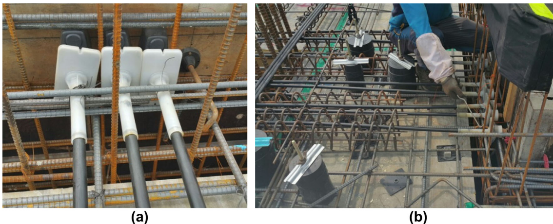
Fig. 13 Applications of developed encapsulated anchor systems. a Stressing end anchors and b fixed end anchors.
