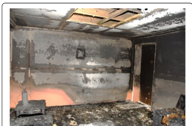
Fig. 4 Varying degree of fire damage to gypsum wallboard-visible damage results
