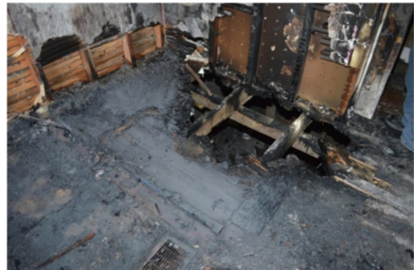
Fig. 10 Photograph of penetration through a floor
