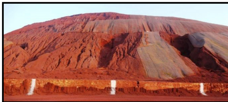
Fig. 6 Photograph of typical failure of coir matting in the iron ore mines of Odisha state
