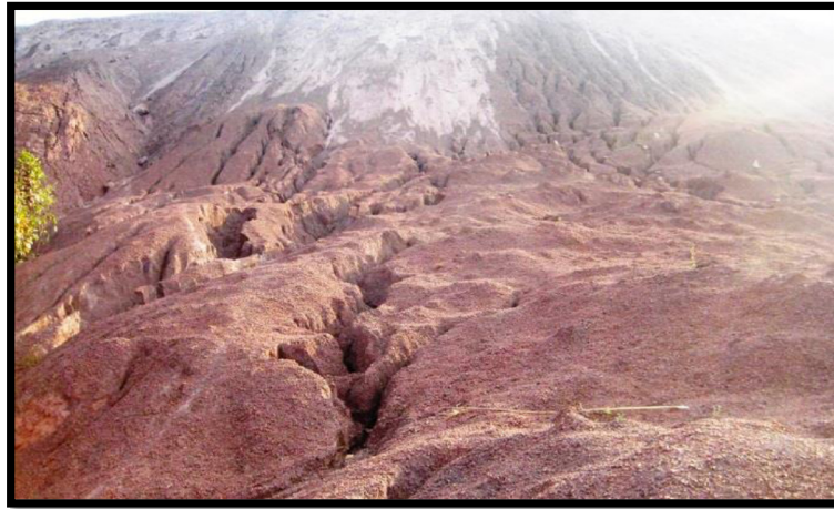
Fig. 1 Slope failure in a subgrade dump of iron ore mines
