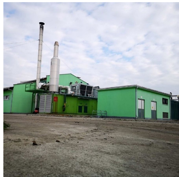
Fig. 2 Biogas plant Buffalo Energy Gold-MG d.o.o. Šamac, Bosnia and Herzegovina [63]
