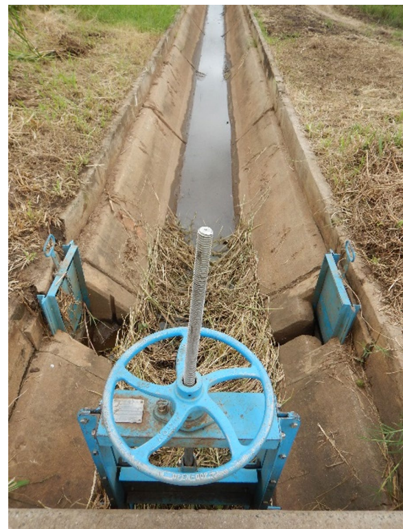
Fig. 8 Mounded grass and debris placed in front of a branching canal slide gate at BVIS to prohibit water flow
