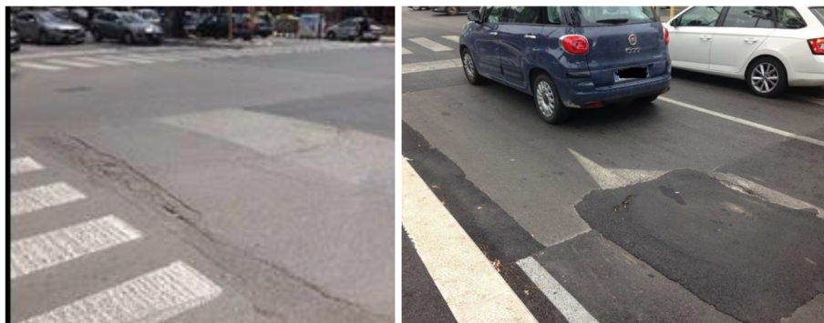
Fig. 3 Example of pavement conditions considered as “poor” conditions (i.e., with cracks, deformations, or potholes on the left; with irregular surface on the right [7].)
