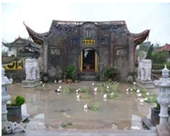
a. Ziguo Temple damaged by wind disaster
