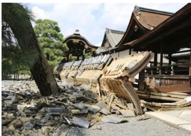
b. Nishihonganji damaged by wind disaster
