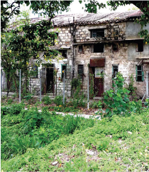
Figure 5 View of the Stone Houses, Kowloon City, Hong Kong before conservation for adaptive reuse (Source: the author).
