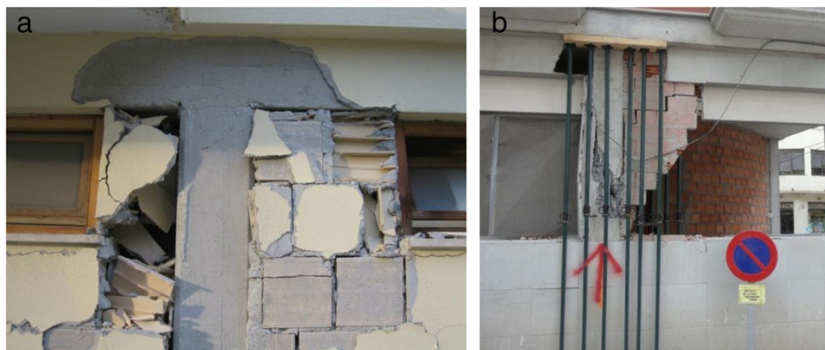
Figure 4 Column failure due to the presence of non-structural elements. Short column effect caused by window openings in residential building. (a) 2009 earthquake in L'Aquila, Italy and (b) 2011 earthquake in Lorca, Spain.
