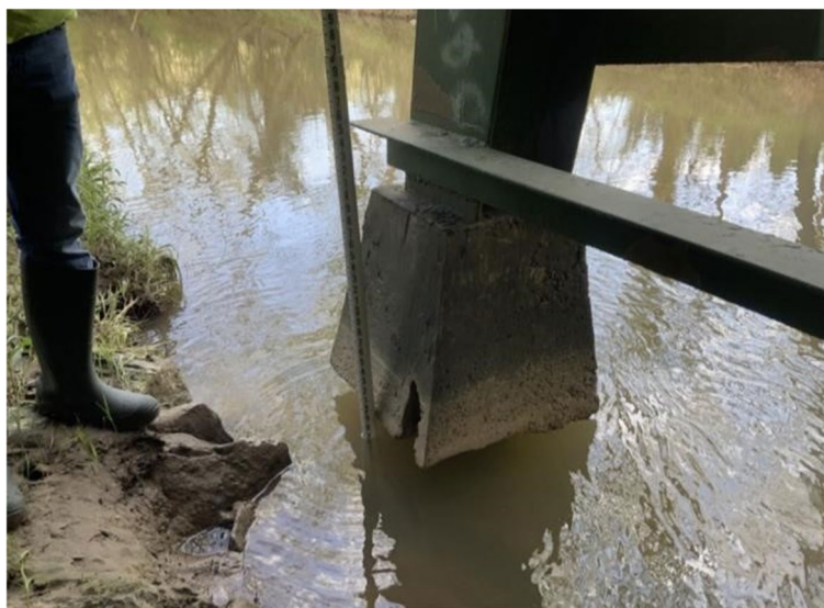
Fig. 1 Scour damage on bridge pile
