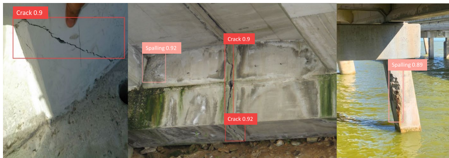
Fig. 7 YOLOv5 performance on concrete bridge defects
