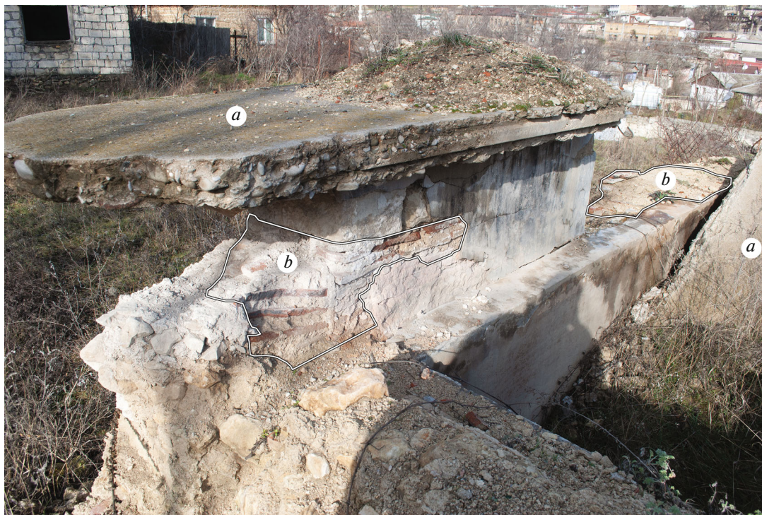
Fig. 5. Hansaray. East building, western wall, inside view: (a) concrete floor slabs; (b) opus mixtum masonry technique.
