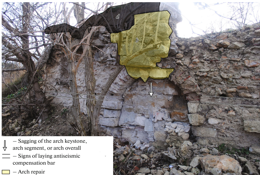
Fig. 4. Hansaray. Eastern structure of presumed Sahib Giray Divan Hall (northern wall). Seismic deformation of plinth-brick arch with a strike 88^\circ : (a) loss of upper central part of plinth-brick arch; (b) plinth arch repair with rubble stone; (c) signs of laying antiseismic compensation bar, duvar-kushak technology; (d) modification of “eastern building” in Soviet period (concrete armored belt).
