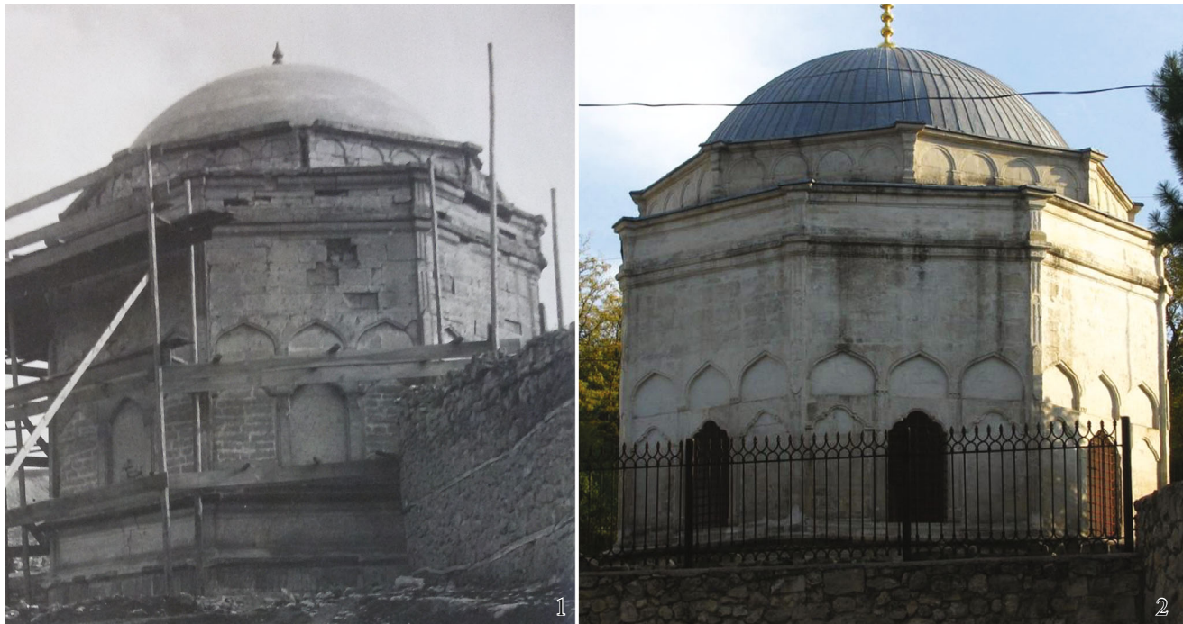
Fig. 6. Dilyary Bikech durbe of Hansaray complex. Face striking 79^\circ . Photo: 1, monument restoration, 1914 (clearly visible are movements of stone blocks in durbe cladding above arches of laid windows, enhanced by skyscraper effect towards building's dome); 2, present state.
