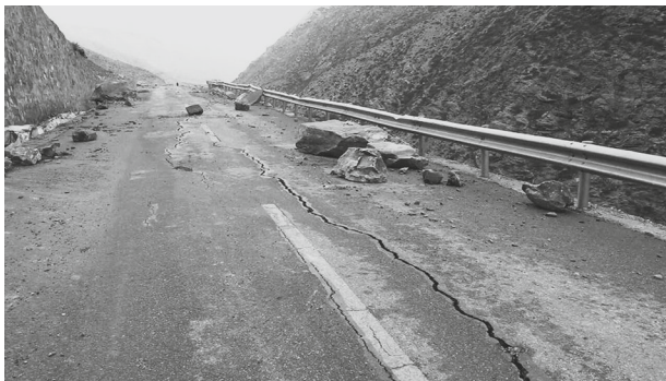
Fig. 5. Vibration cracks on road in High Himalayas.
