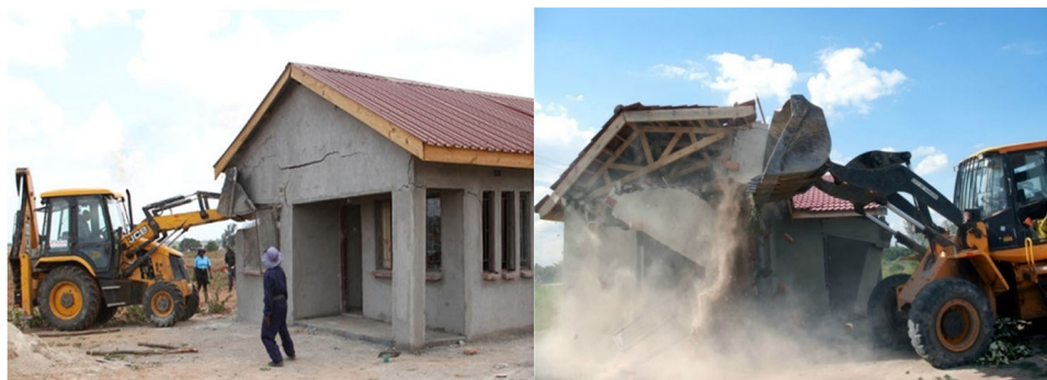
Fig. 4 Demolitions of houses built on illegal land in Harare, Zimbabwe. This figure is not covered by the Creative Commons Attribution 4.0 International License. Reproduced with permission of NewsZimbabwe; copyright © NewsZimbabwe, all rights reserved.
