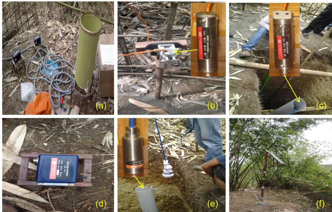
Fig. 13 View of geosensors and solar panel installed at Karshingsa landslide prone area: a raingauge, b tiltmeter, c in-place inclinometer, d crackmeter, e piezometer, and f solar panel
