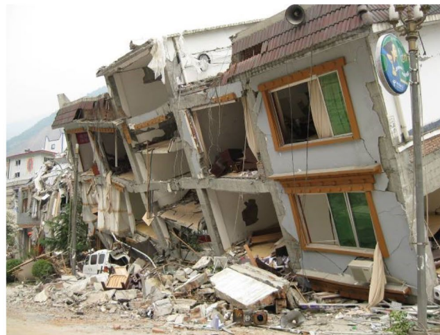
(e) Complete failure of the bottom layer of the structure
