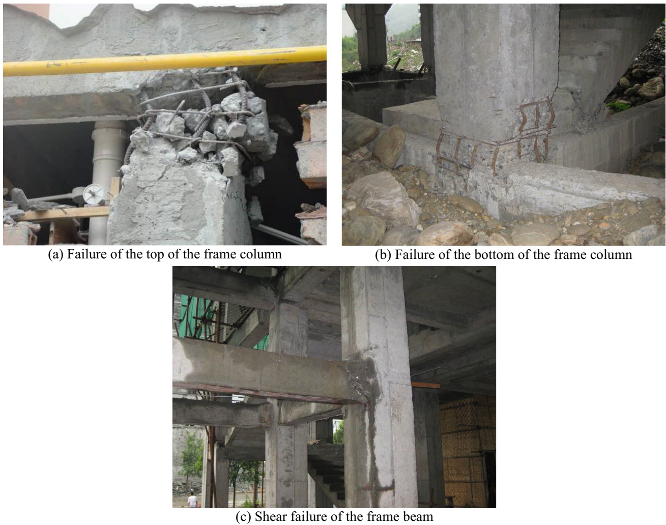
Fig. 4 Failure of typical structural components
