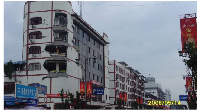
(b) Cracking and local collapse of infill walls
