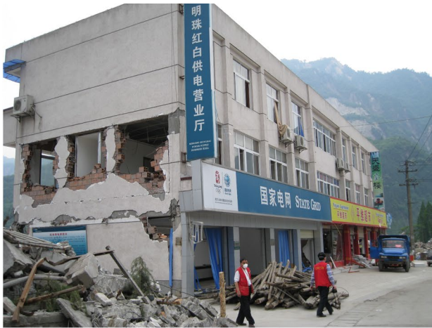
(a) Partial failure of infill wall
