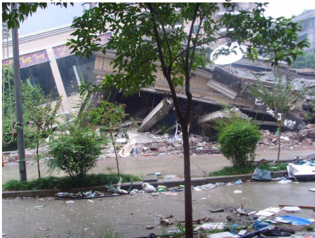
(c) Overall failure of a single structure
