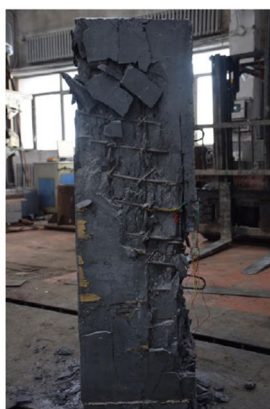
(c) Incline failure plane of specimens
