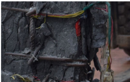
(b) Fracture of rectilinear ties
