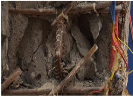
(a) Buckling of longitudinal reinforcements
