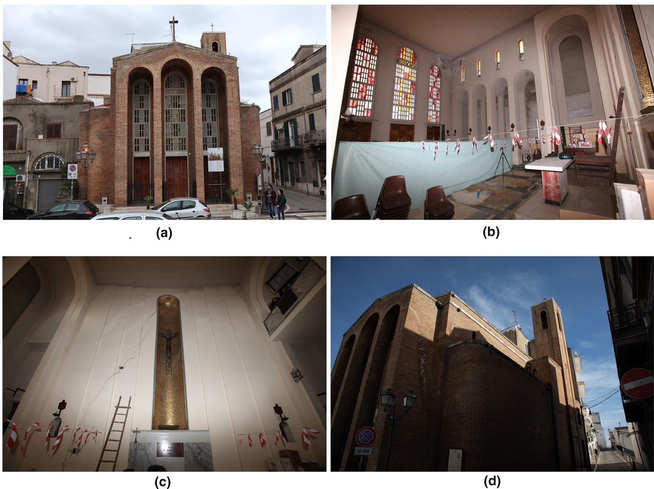
Fig. 1 a Frontal view of San Rocco Church, b internal view looking at the main façade, c diagonal crack interesting the wall behind the altar, and d bell tower
