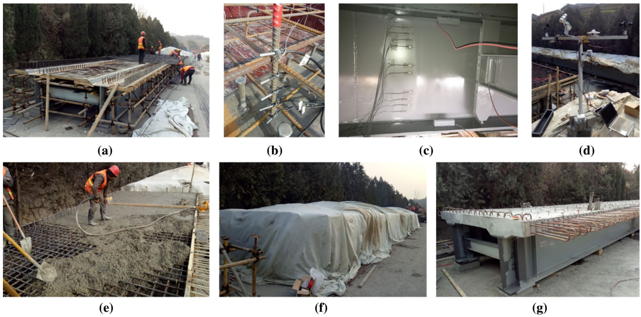
Fig. 4 Experimental photographs: a reinforcement assembly, b temperature sensors arrangement in concrete deck, c temperature sensors arrangement in steel girder, d mobile weather station, e concrete cast, f concrete curing with asbestos cloth and g constructed composite girder
