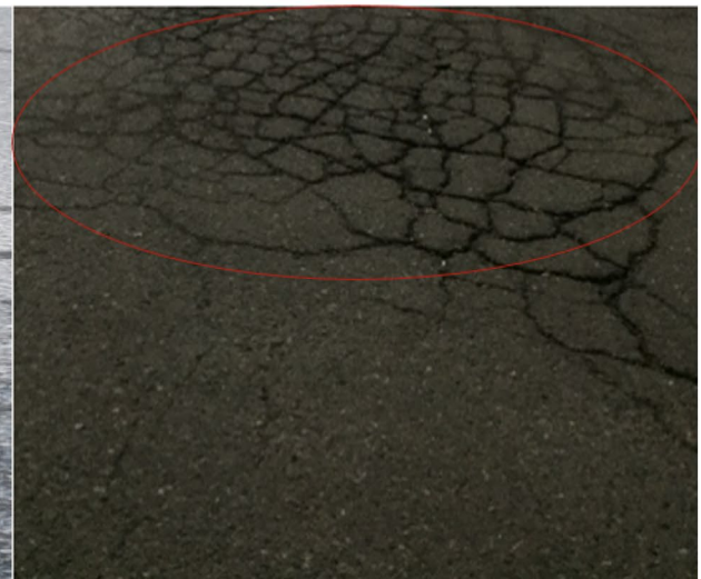
(e) Fatigue Cracking
