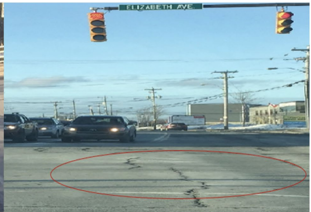
(b) Transverse Cracking
