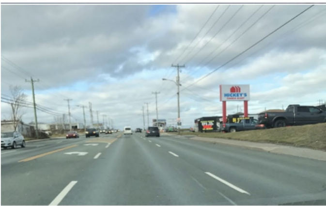
(c) Structural Rutting
