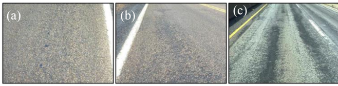
Fig. 2. Raveling classification in GDOT [2] (a) Severity Level 1, (b) Severity Level 2, and (c) Severity Level 3.
