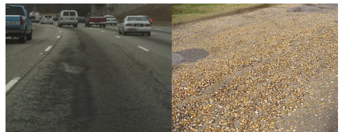
Fig. 1. Raveling on interstate highway and non-interstate road.
