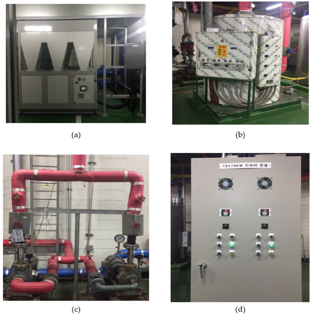
Fig. 8 On-site photograph of comprehensive BEMS construction/ demonstration facility at site #1, a Air heat pump; b Electric boiler; c Cold and hot water circulation pump; d inverter
