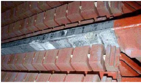
Fig. 1 A stator winding damaged from vibration abrasion
