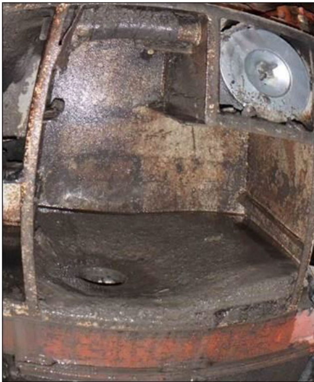
Fig. 2 Dry dust collector box that has been converted to the wet box.
