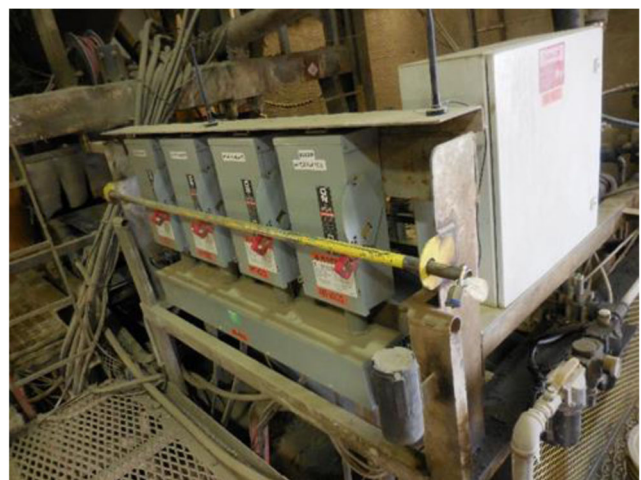
Fig. 2 Locked out disconnect panel
