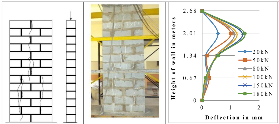
Fig. 6 Views of failure patterns and distribution of lateral deflection along the height at various stages of loading of wall no. 2 (HCB-200-A2)
