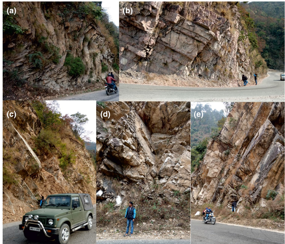
Fig. 2 Unstable conditions favouring structurally controlled failures at road cut slopes along NH-58 from Kaliyasaur to Rudraprayag. a Extensively folded discontinuities showing a high stress regime and toppling failure conditions (slope 2); b large persistent discontinuities showing daylight conditions favouring planar failure (slope 3); c rock mass with large and persistent discontinuities prone to the planar and wedge mode of failure (slope 4); d blocky and highly fractured rock mass forming wedge failure (slope 5); e persistent discontinuities forming a favourable condition for the planar mode of failure (slope 7)
