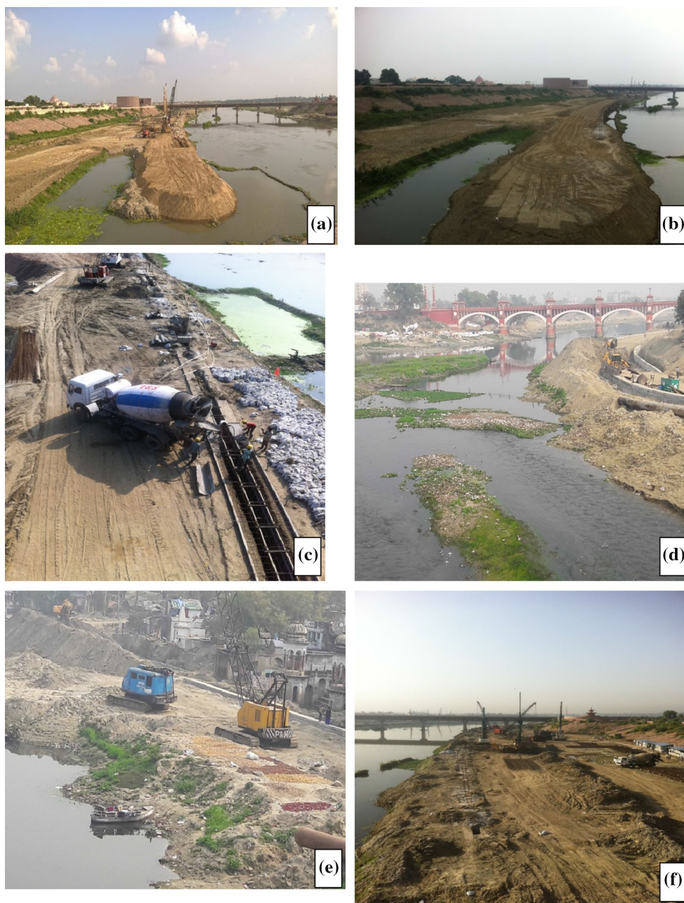
Fig. 3 Channel straightening and construction of diaphragm walls across the Gomti River banks
