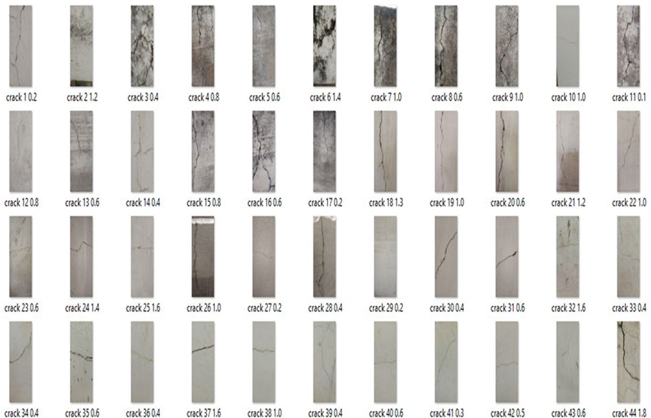
Fig. 7 Images collected using a crack microscope
