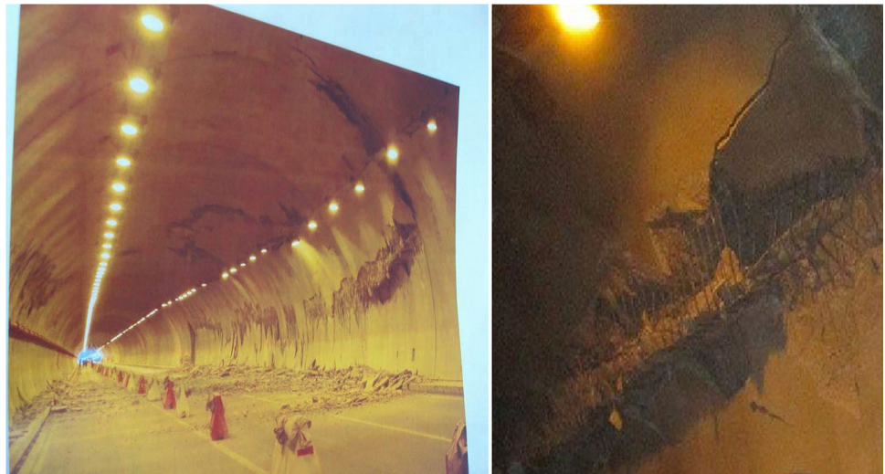
Fig. 5 The state of place of the structure after the collapse (left tunnel liner damage)
