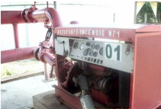
Fig. 1 View of fire pump unit No. 1 and 3
