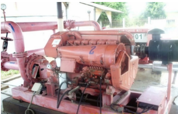
Fig. 2 View of fire pump unit No. 2
