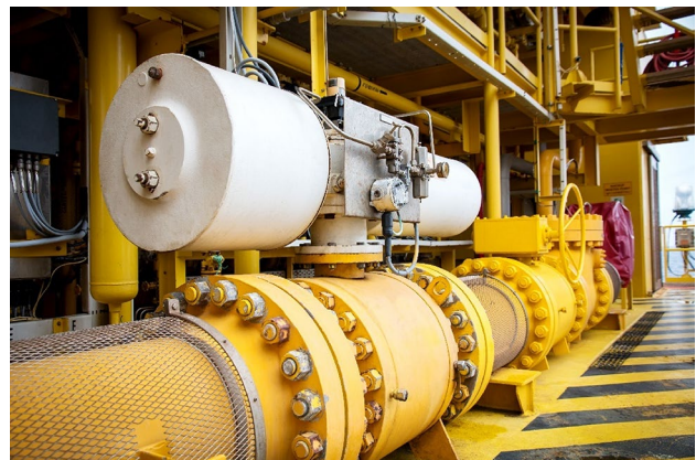
Fig. 3 An ESD valve is installed in the gas piping system. (Courtesy: Shutterstock)
